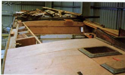
'Before and after...' Fortunately not every refit need be as comprehensive as that required on Lady of the Sea . However even a task this daunting is entirely feasible provided that proper planning and budgetary controls are put in place. Remember that time usually equals money, in refits as anywhere else. If you 'need' a job to be rushed, then the final bill is likely to be considerably higher than if you had allowed more time for the work to be carried out
